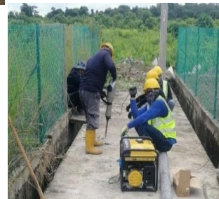
TM CNC LITE - TELCO INFRASTRUCTURE
